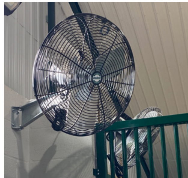
▲ Fans for Ventilation
